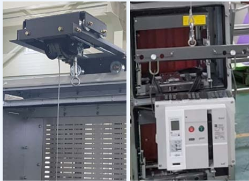
Hoist mounted on switchgear
