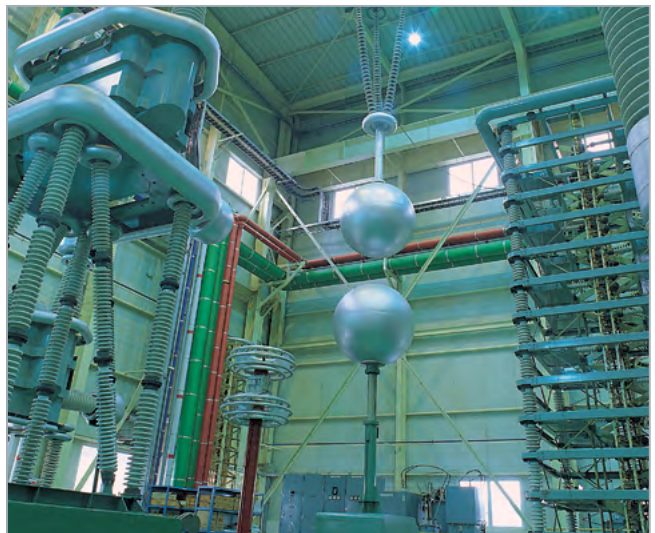
High Voltage Test | Impulse Test
